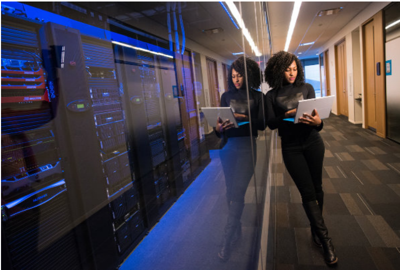
An employee checking on a data center. Photo Courtesy of Christina Morillo
